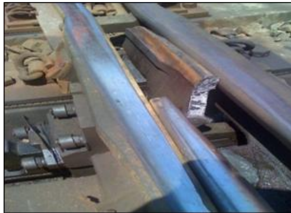
Figure 1: Point rail fatigue fracture of movable-point frog
