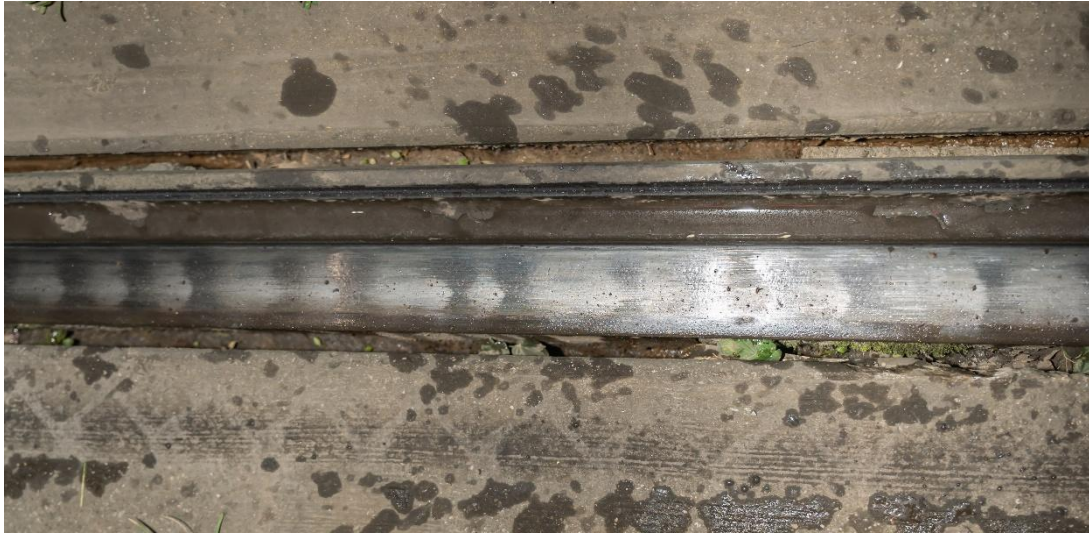
Figure 2: Example of corrugation severeness at selected track location
