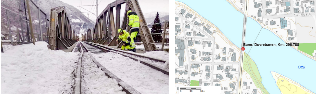
Figure 1: Railway bridge over the Otta river with visible track alignment and inspection work following the 2025 damage event [16] (left). Km 296.788 along the Dovre Line [4] (right).
