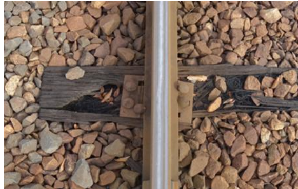
Figure 7: Rotting of a wood sleeper [3].
