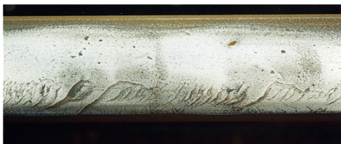
(a) Severe head checks on rail surface
