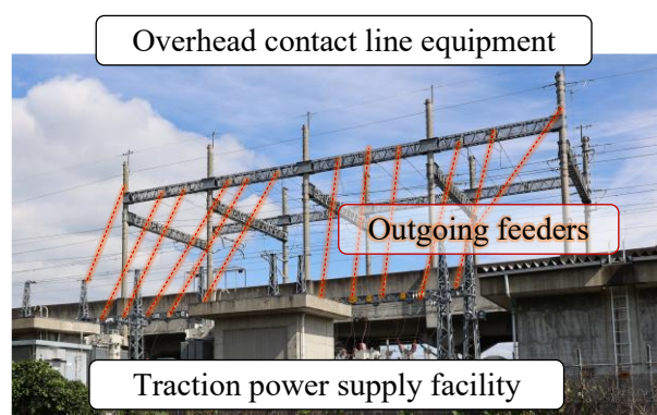
Figure 1: Example of Shinkansen overhead contact line equipment at a traction power supply facility.
