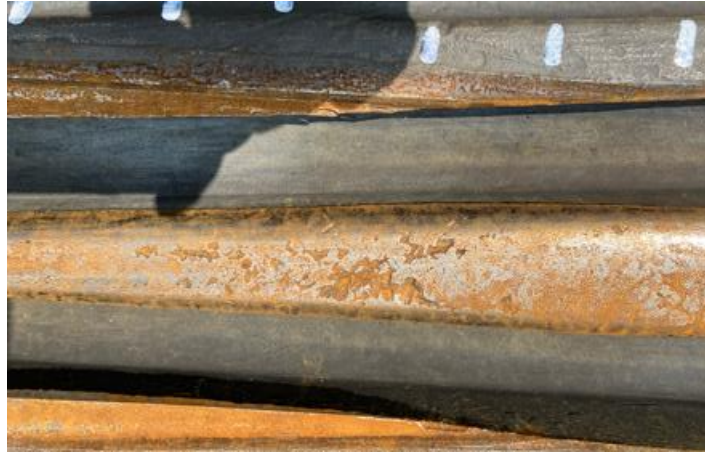
Figure 1: Defect appearing on fixed crossing.
