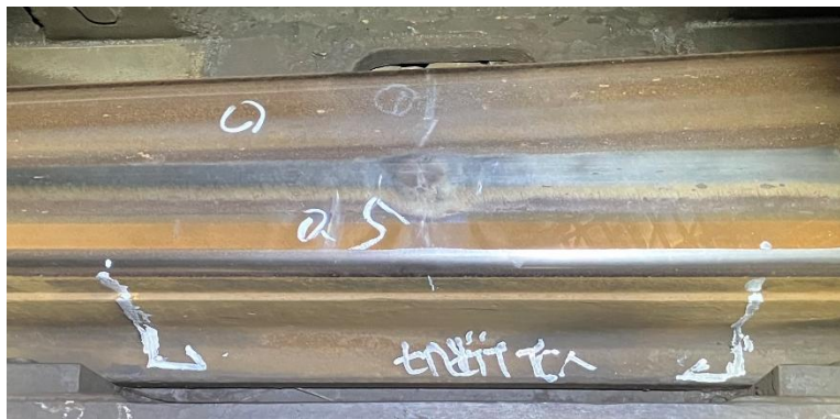
Figure 2: Defect on swing-nose crossing.
